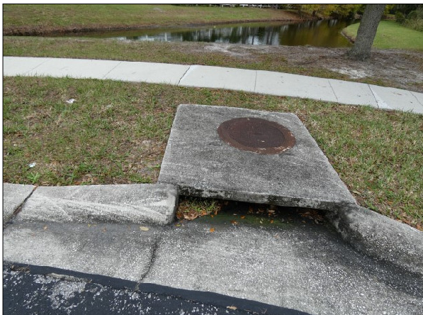
Stormwater Drainage Curb Inlet
